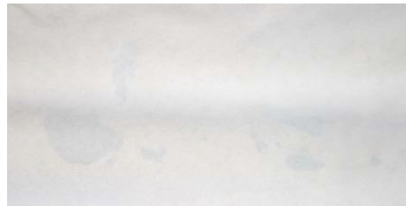
Photograph 4. Fabric Discolouration Due to the Coating Failure
